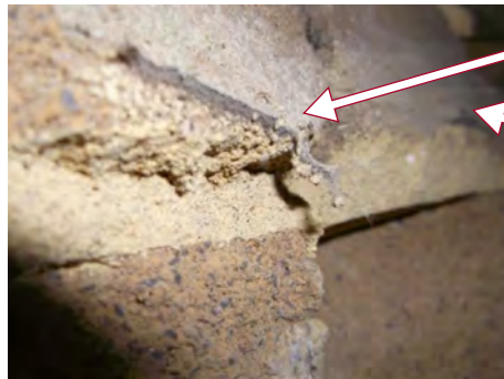
Figure A5.9 Remnants of asbestos on materials
