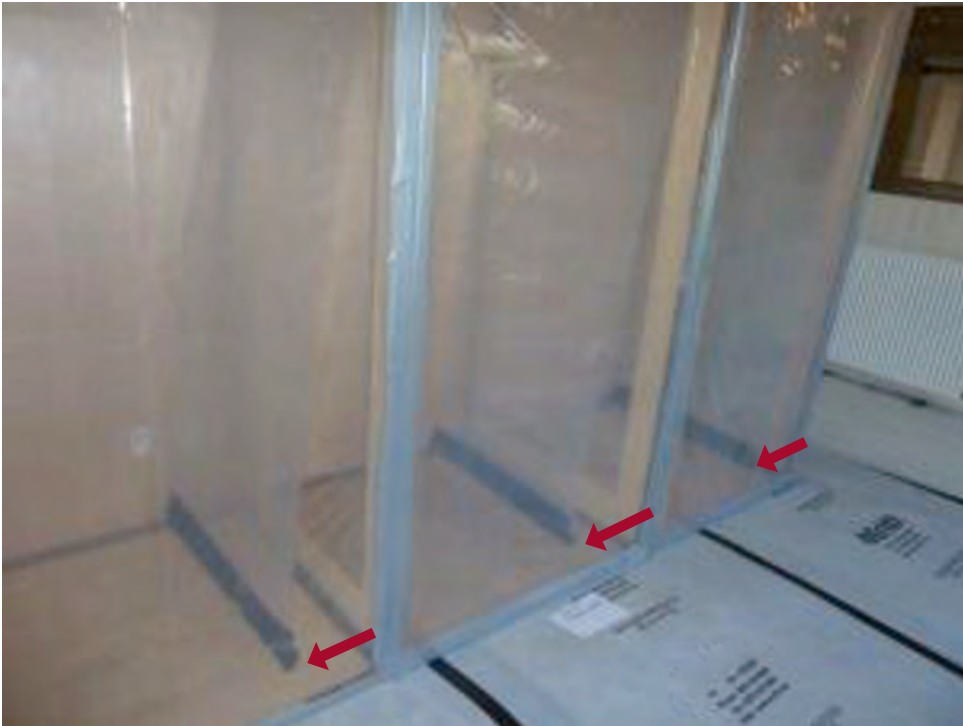
Figure 5.7 Airlock door flap deflection of 200–250 mm in chambers 2 and 3 at the base of the flap (see arrows) indicates that the NPU is extracting 1000m 3 /hr and enclosure internal negative pressure is –5 Pascals (see Asbestos enclosure ventilation research ) 38
